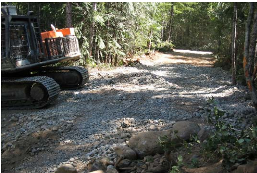
Photo 7. Spur road constructed to access site near Second Lake outlet, Nanaimo River.
