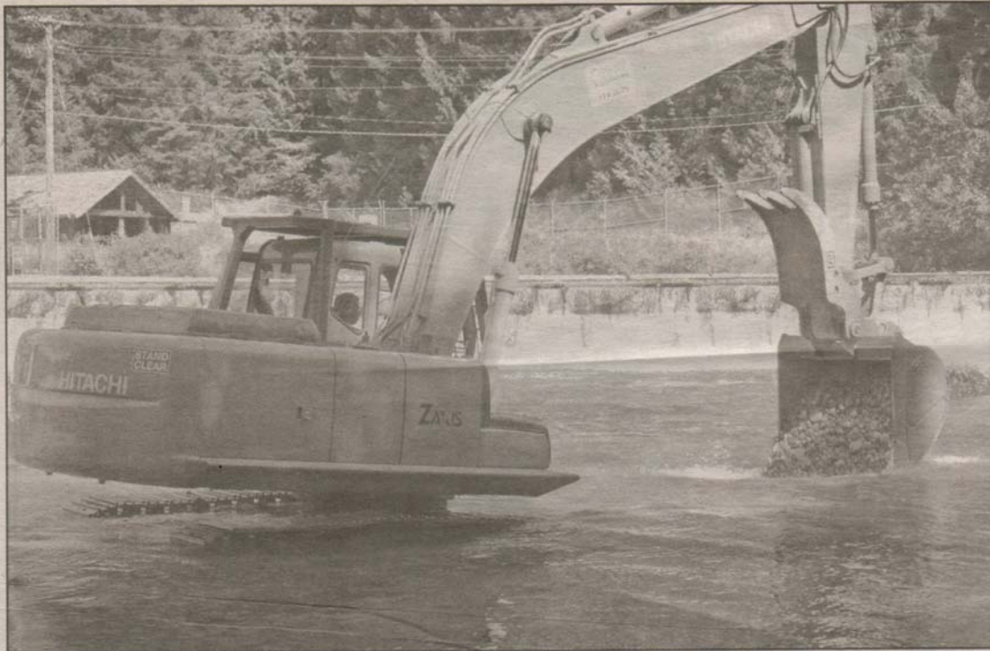
A FISH-SAFE EXCAVATOR placed gravel above Stotan Falls and below the diversion dam. The $37,000 enhancement will provide about a 25 per cent increase in spawning habitat.
