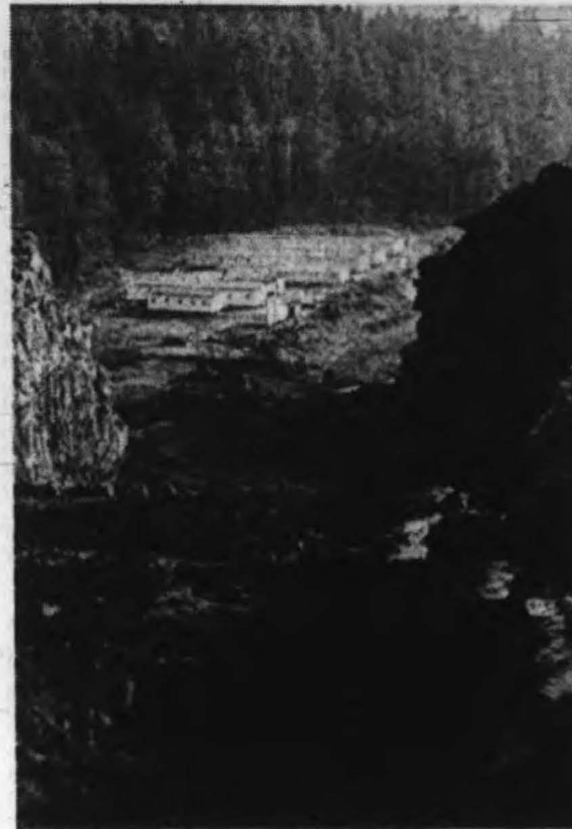
View from the mouth of the new tunnel looking down towards a construction camp at Jordan River. The penstocks will be laid down the excavated slope to the new power house site.—(B.C. Hydro)
