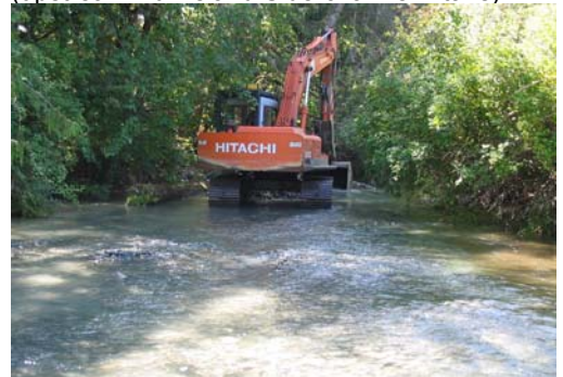
6. Gravel pad creation by excavator at Site 3 (opposite Bull Island S/C outlet).
