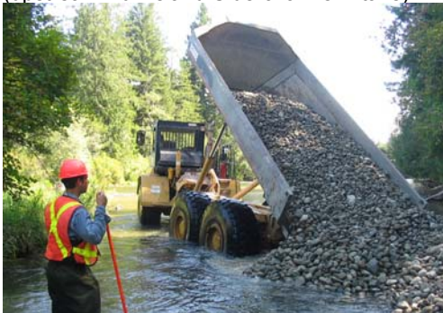
5. Gravel placement by articulated hauler at Site 3 (opposite Bull Island S/C outlet).
